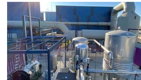
Thermal Hydrolysis Plant
