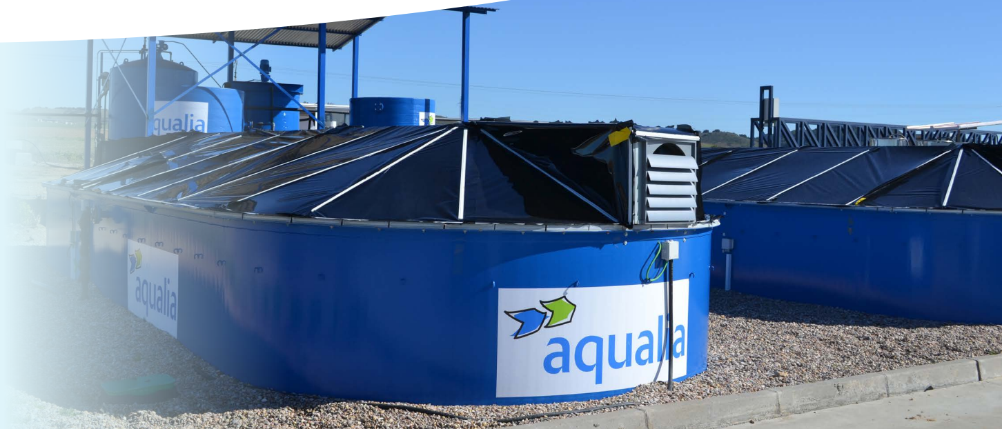
Deep Purple Project at the Wastewater Treatment Plant in Toledo (Spain).
