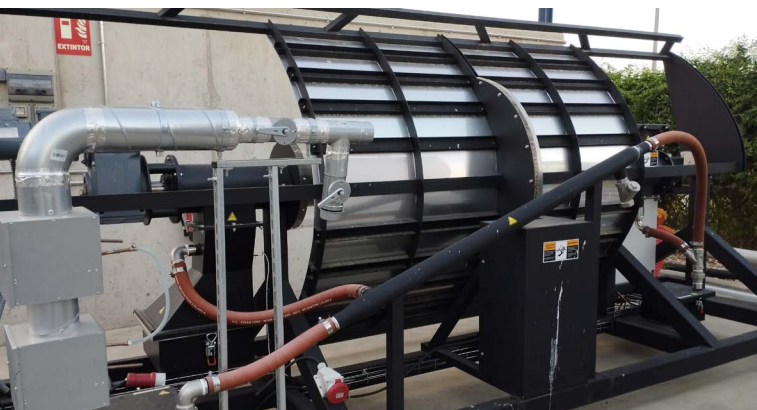
Solar tubular dryer at Las Dehesas, Madrid (Spain).
